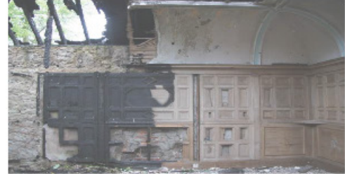
inside the north annex with burnt wood panelling and some painted decoration still visible on the curved ceiling above below the charred timbers of the roof structure
