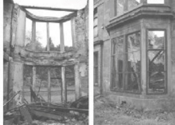
view west looking out through the projecting bay, note the nochas in the stonework between the floors where the joist ends were fitted prior to the fire
